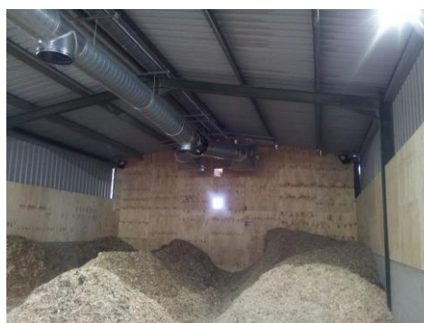
Above – The Ducting at GWR Ltd
