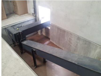
The auger linked to the walking floor wood chip delivery system and the Viessmann boiler.
