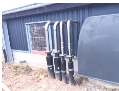
Above – The district pipe supplying the heat into the poultry sheds, before being insulated.
