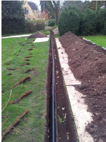
Above and right: District pipe installed within a trench and a fan heater fitted within the greenhouse.
