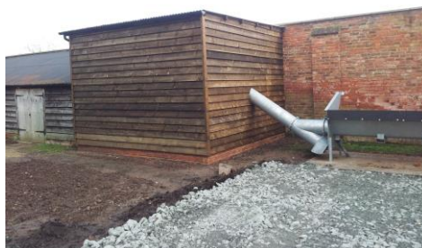
Above: The wood chip hopper and chip shifter before landscaping
