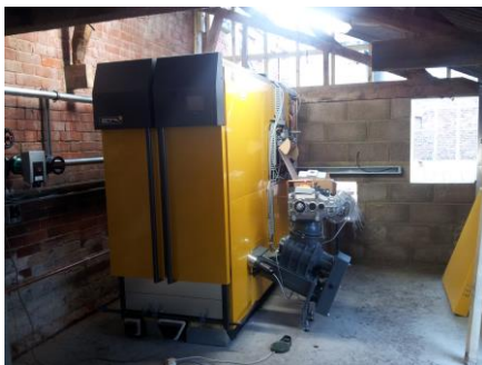
The boiler and burner which connects the fuel store - pre commissioning.
