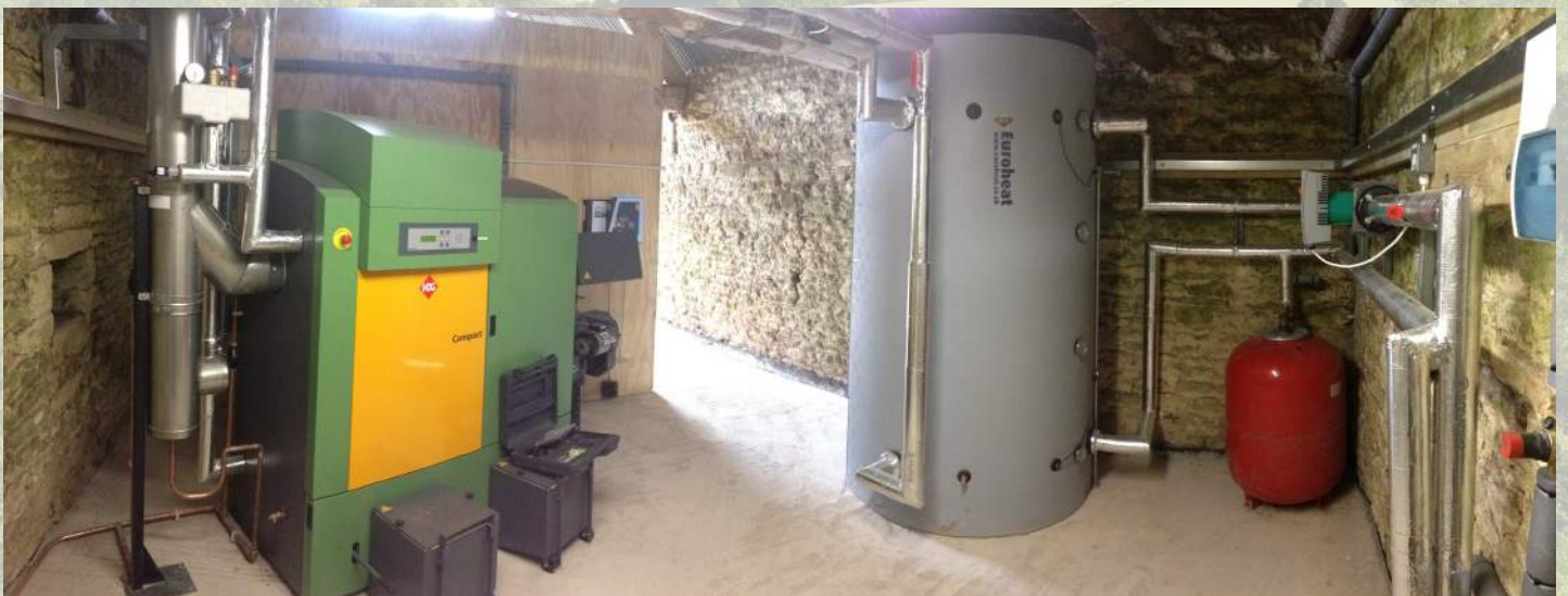
Within the boiler shed at Lower House.
