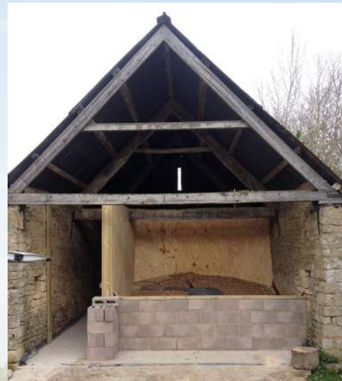
The chip store and boiler shed for the boiler.
