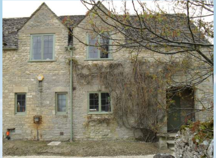
The second heated property at Lower House.
