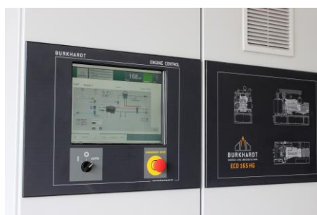
Above – Control interface for the CHP, operated both manually and remotely.
