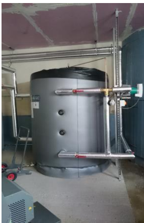
The 4,000 litre buffer tank.
