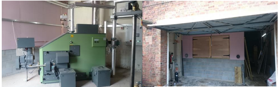
The plant room – Internal & Wood Chip Store
